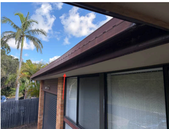
Areas where roof has bowed over window openings.
