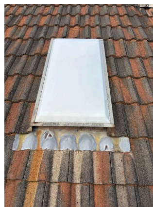
Skylight that leaks
