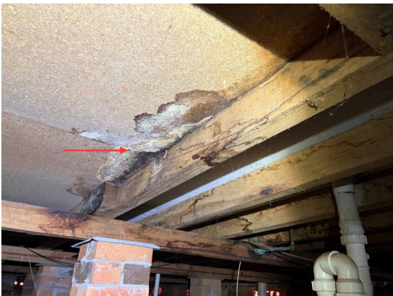
Water leaking onto flooring below shower.
