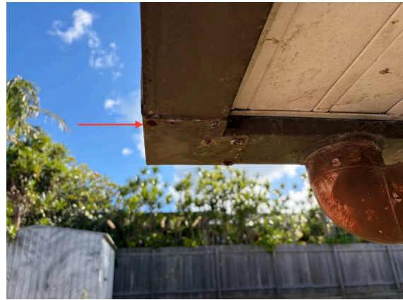
Areas of rust
