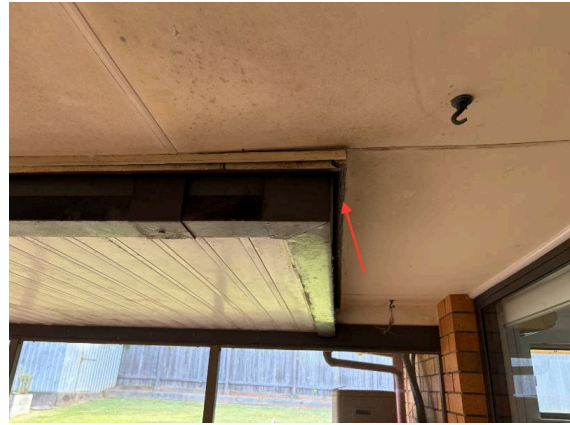
Areas where patio is susceptible of leaking.
