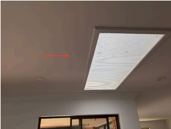
Area where skylight leaks onto the ceiling
