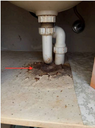
Water damaged shelving
