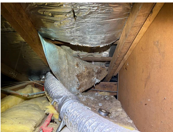
As seen from the roof void, area where water leaks from sarking out of place.
